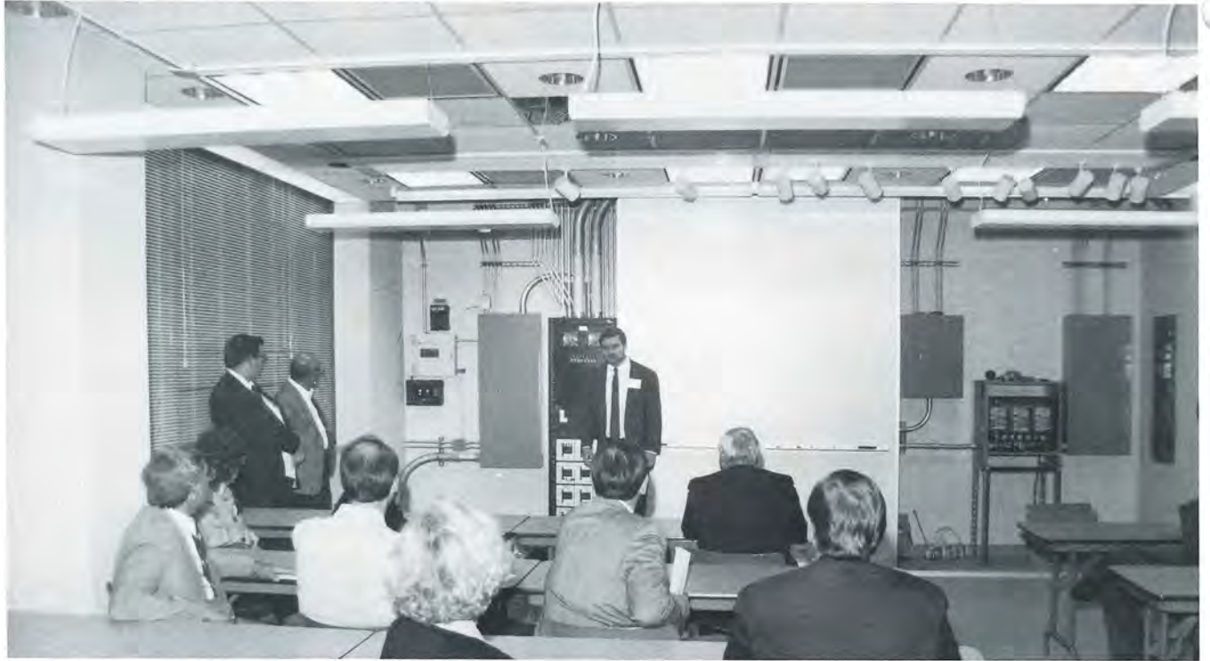
Clarence Waters, asst. prof. AE & CnS, explains functions of the newly completed lighting lab in Seaton Hall, following dedication ceremonies. It will be used for research, teaching, and seminars.
