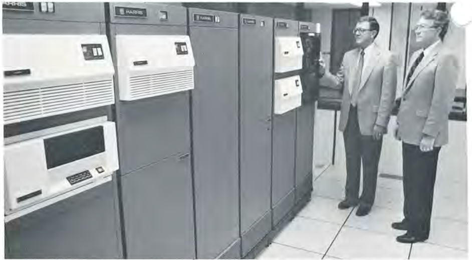
Harris 800 super-minicomputers were major additions in $1 million expansion of computing facilities. From left are Dean Donald Rathbone and Associate Dean Kenneth Gowdy.
