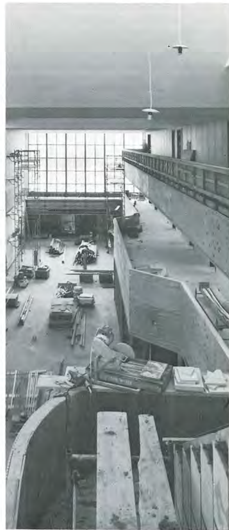
Construction continues on the main lobby area of Durland, Phase II. The lobby extends through the building. Balconies open onto the lobby from each of the upper stories, adding a pleasant airiness. A student study lounge will overlook the lobby from the south end of the building. Aesthetic appeal will be heightened with decorative stonework on stairwells and the use of bright colors on walls.
