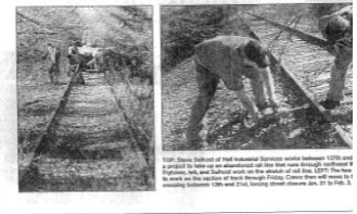
Carl Ligon, president of the Patrons Neighborhood Association, is working on the railroad track between 17th and 20th streets. He and his volunteers are clearing the track of debris and preparing it for a trail.
