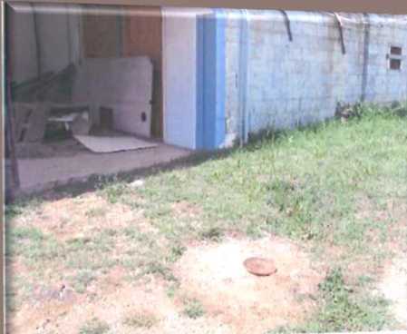
Photo #15 View northeast of fill port and vent pipe for the 10,000-gallon diesel tank.
