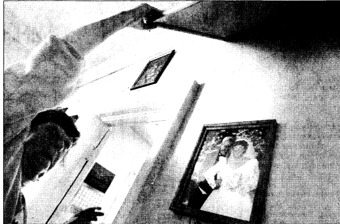
Nellie Culter displayed a crack in the living room wall that she deduces is from various shifts in the foundation of her house because of the poor soil quality of the land under her home at 316 S. Keeler, directly west of the former site of Chemical Commodities, Inc.
